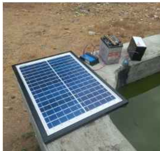
Gambar 4. Alat Monitoring Water Turbidity Berbasis PLTS
